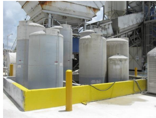
Plastic Admix Tanks in Containment
