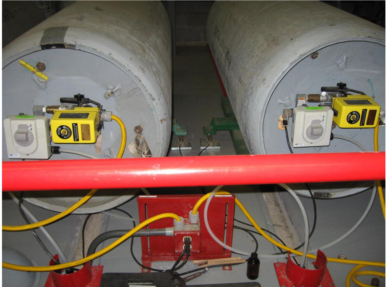
1-ton chlorine gas cylinders
