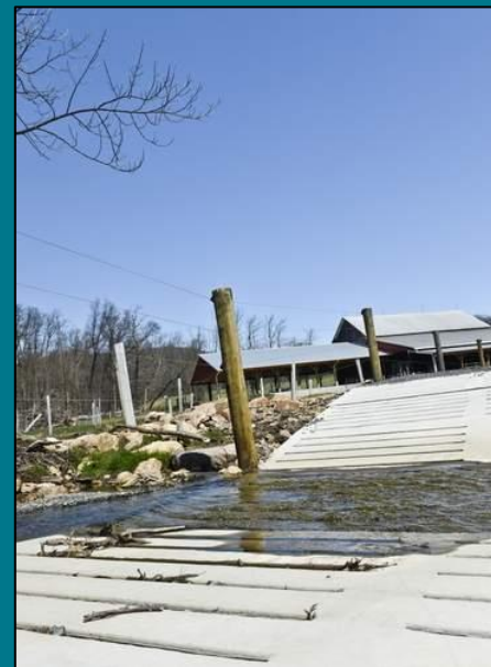
The newly engineered cattle path at Furnace Stream Farm in Windsor Township protect their water resources. Berks Nature and Stroud Water Research Center and other groups are working with farmers in the region to protect water resources and reducing pollutants on farms.
